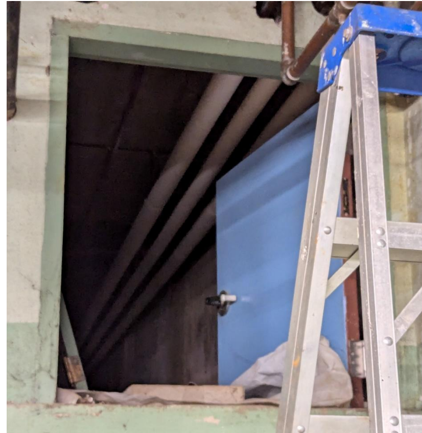
A partial height door providing access to a mechanical system crawl space that serves a portion of the original school.
