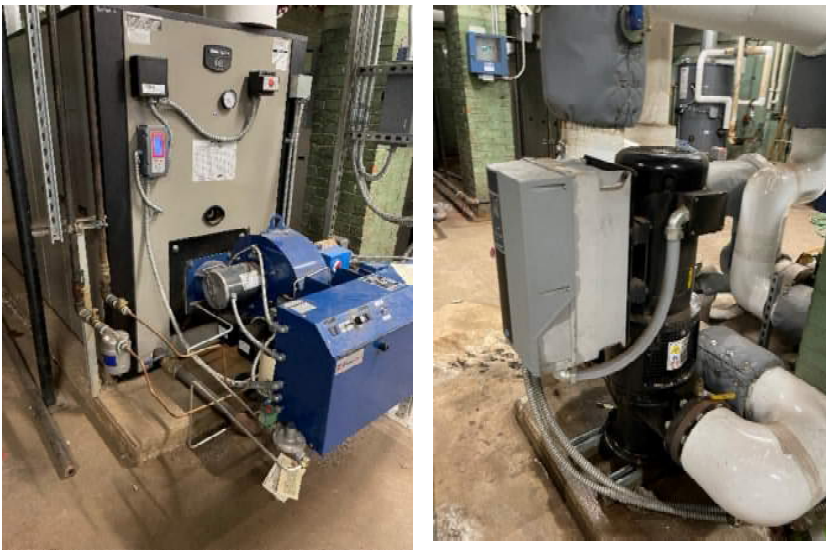
A view of the hot water heater (left) and circulating pumps (right).
