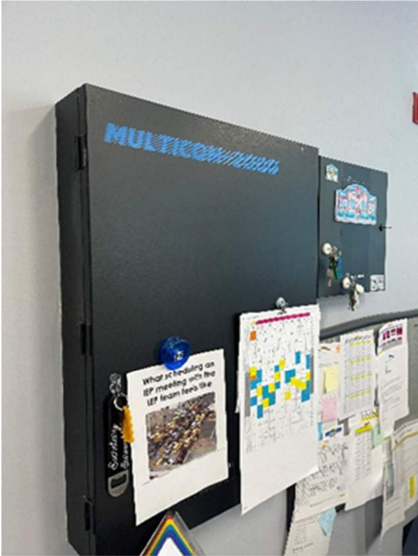
Multicom PA System in the Administration Suite
