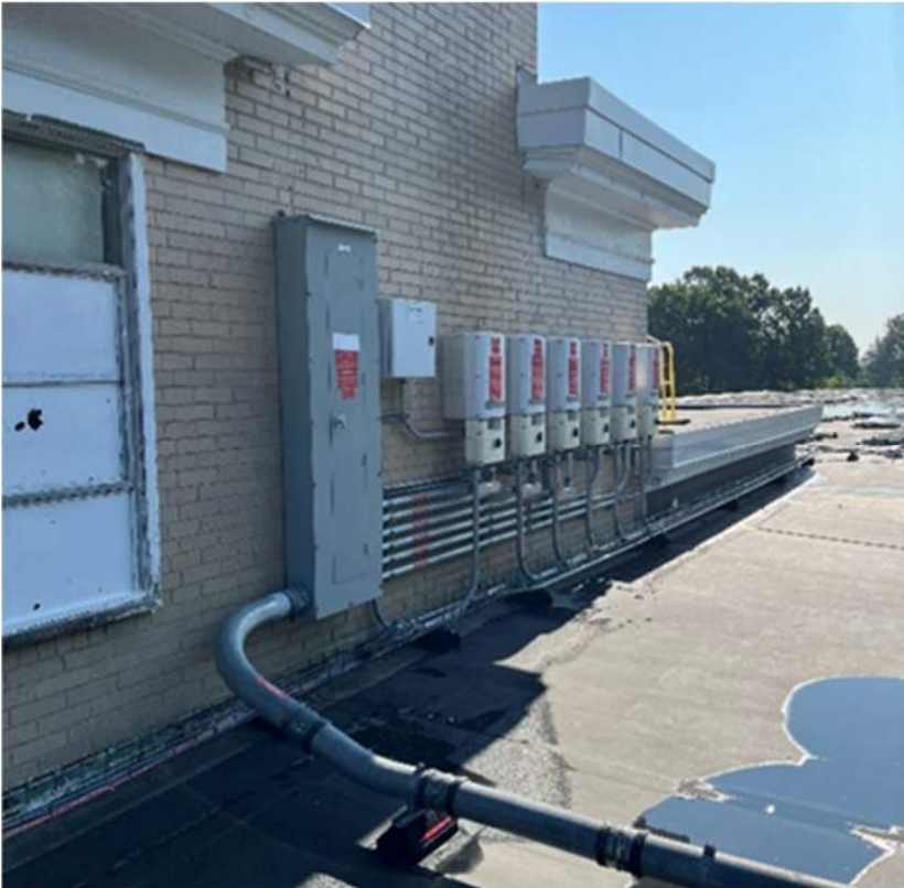
Roof top 480V Solar Equipment.
