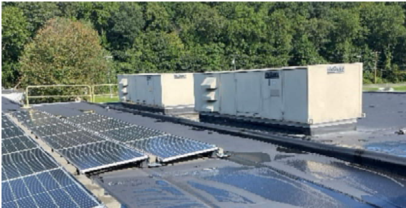
A view of a typical rooftop unit serving the gymnasium.
