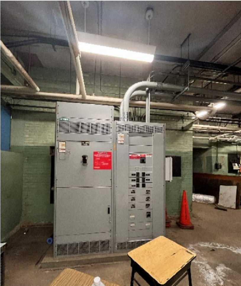
Main switchboard in basement boiler room.
