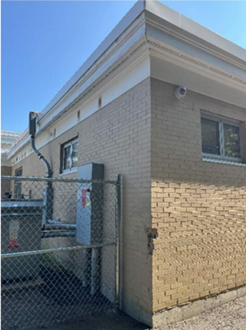
Solar PV system equipment on grade.
