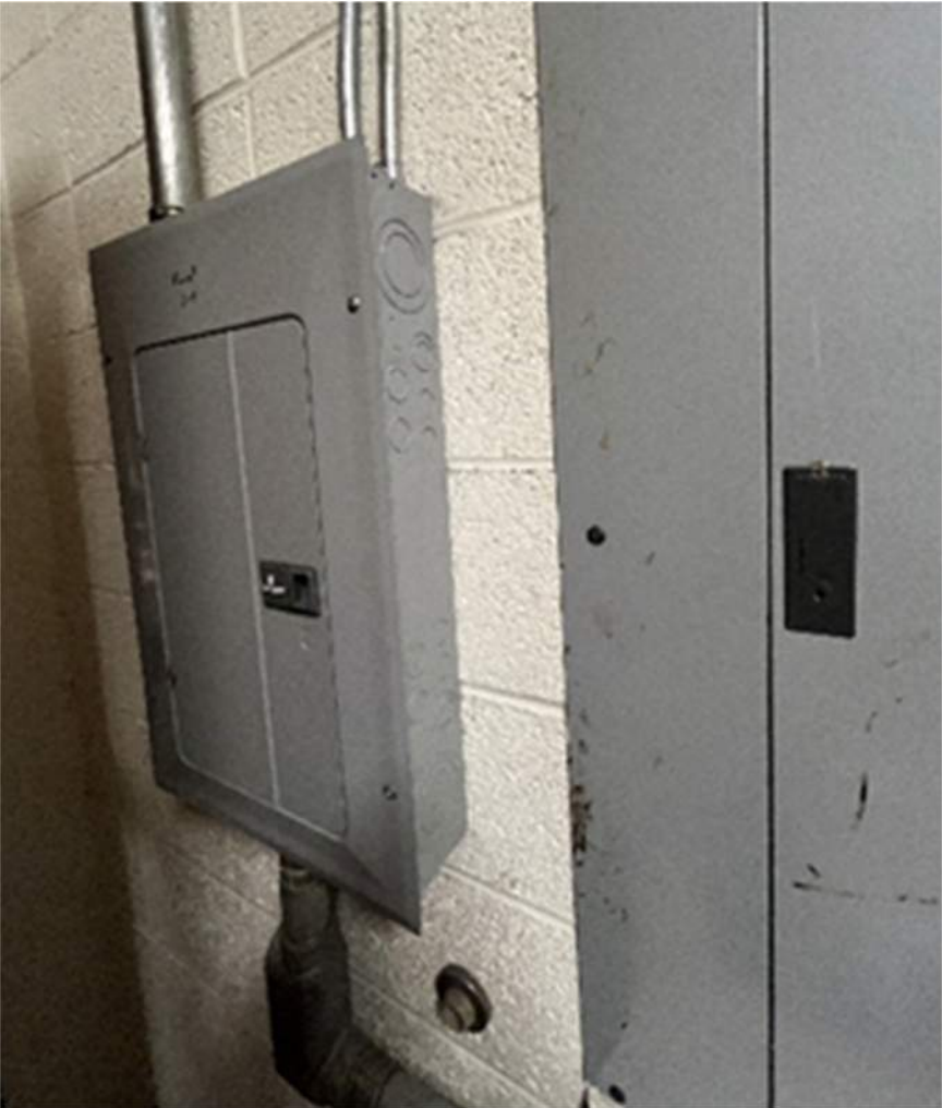
Electrical Distribution in MDF Room
