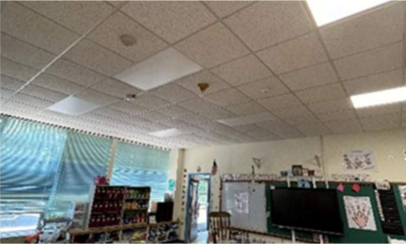
Typical Classroom Lighting
