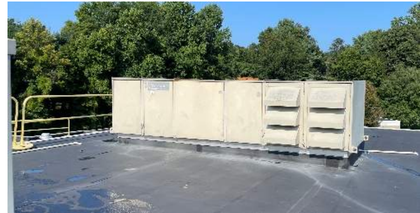
Rooftop units serving the cafeteria.
