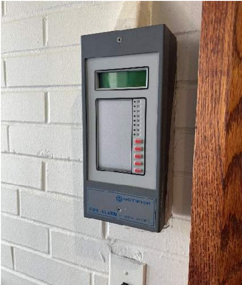
Inoperable (abandoned) fire alarm annunciator panel in the entry vestibule.
