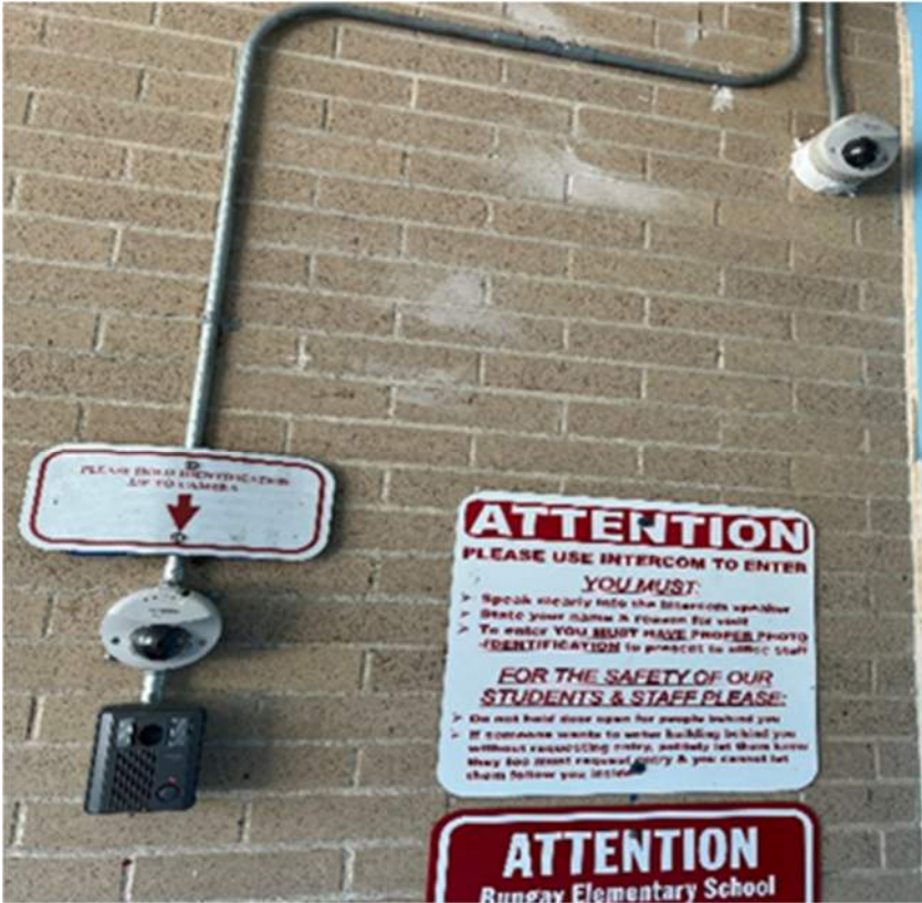
Security camera at the Building Main Entrance
