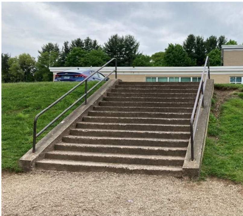
Existing exterior concrete stairs leading from the school level to the lower fields.
