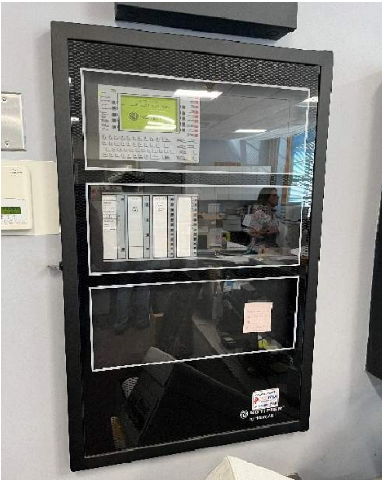
Notifier Fire Alarm Control Panel in the Administration Suite.
