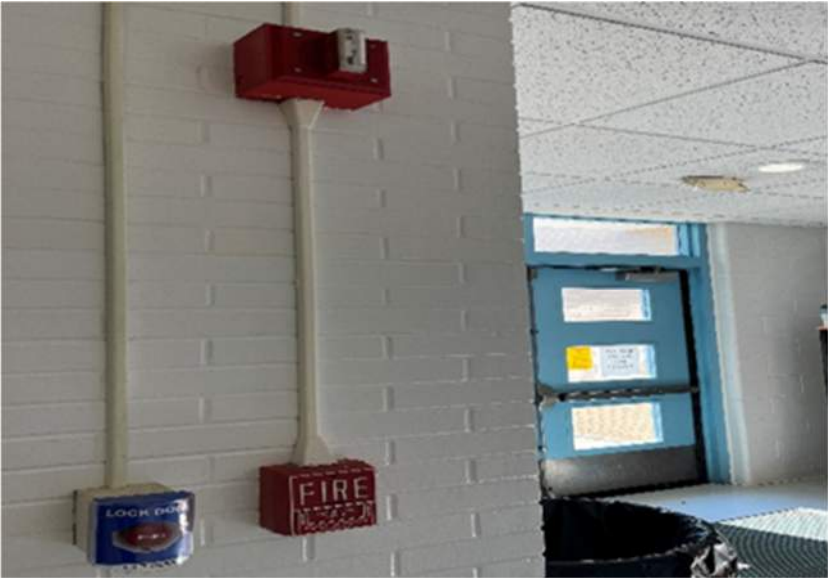
Fire Alarm manual pull station and strobe in a corridor
