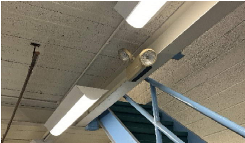
Typical self-contained battery backed emergency lighting units with twin heads in a storage space.
