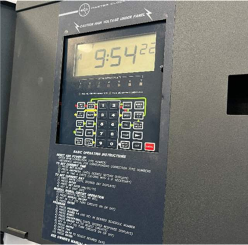
Notifier clock system in the Administration Suite.
