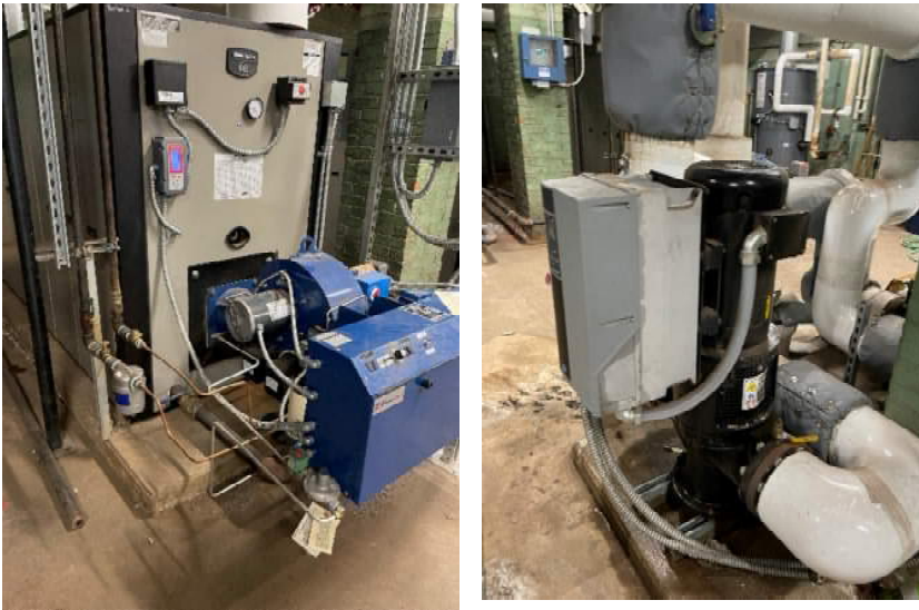
A view of the hot water heater (left) and circulating pumps (right).
