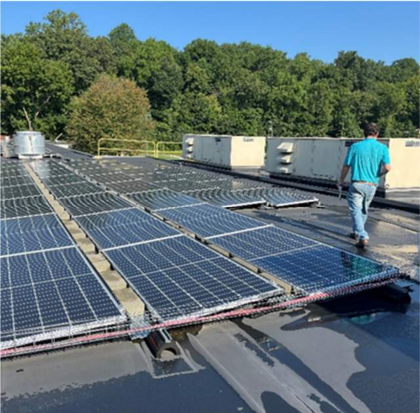
Roof top photovoltaic system.
