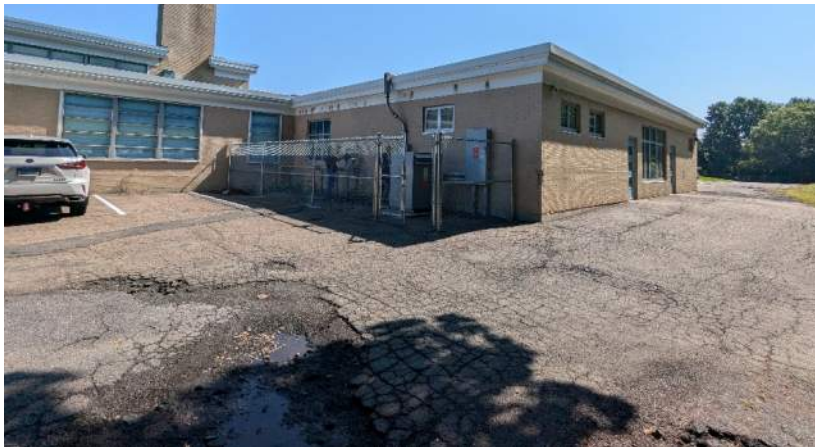
Visible surface deterioration of the existing south access drive and parking
