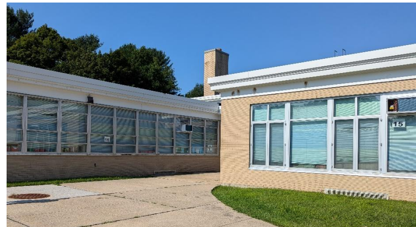
Storefront glazing utilized during the 1996 improvements project at the right of the image with the older pattern storefront windows used in classrooms on the left (above).
