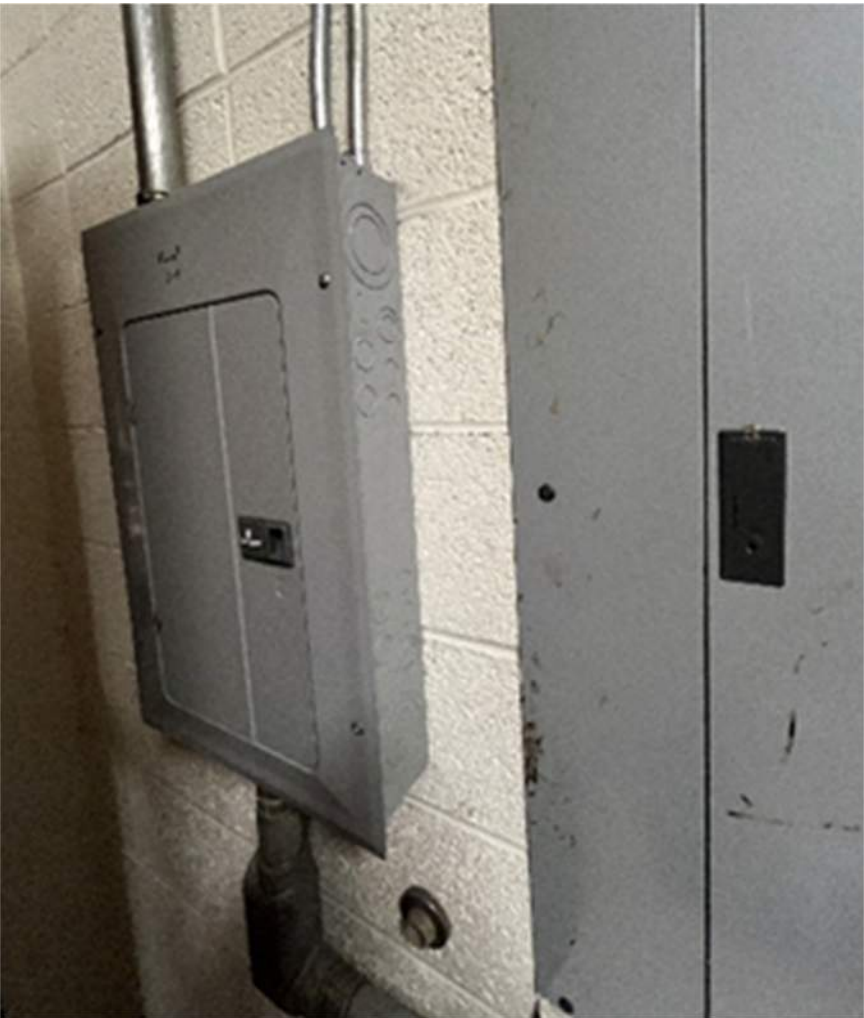
Electrical Distribution in MDF Room
